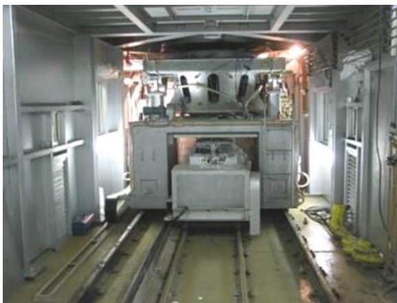
Fig.6 No.3 engineering scale furnace (Capacity: 430kg-Fe/batch)
