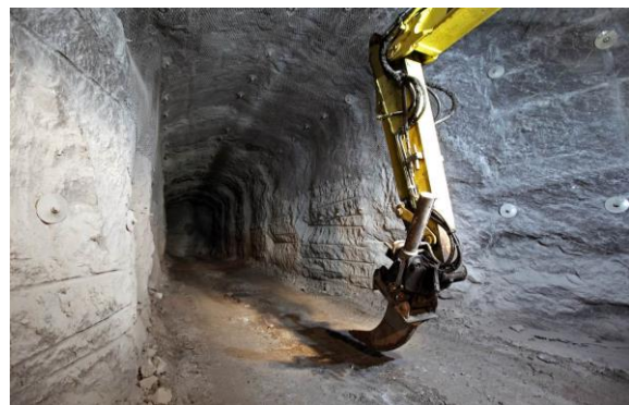
Fig. 6: A photo of the demonstration tunnel 2 from Posiva Oy’s website [18]. It shows a dry condition in the tunnel.
